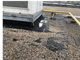
Near Rooftop Mechanical Units
