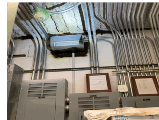
Electrical Panel Room
