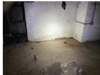
Gas Meter Room
