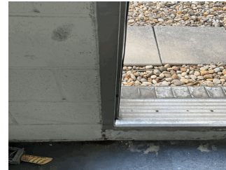
Bulkhead BH1 (deteriorated weatherstripping)
