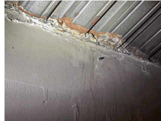
Mechanical Room above Auditorium
