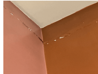
Outside Mechanical Room Stair F
