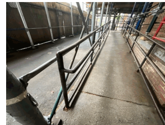
Exit 2 Ramp (loose)
