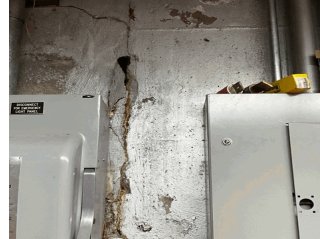
Electrical Panel Room shown, also South Fan Room
