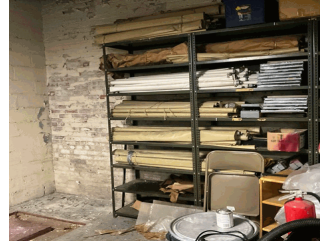
Mechanical Room near Stair A shown, also at Boiler Pit
