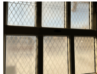
Bulkhead BH (clouded glazing)
