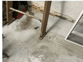
Boiler Room Mechanical Area shown, also Boiler Room, Oil Tank Room, Gas Meter Room, and Stair in Custodians Bathroom
