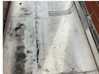
Roof 1 near Bulkhead BH2 (delaminating)
