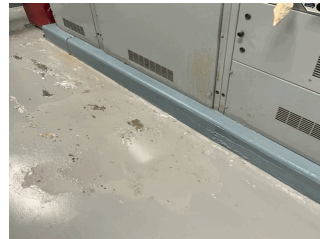
Electrical Panel Room
