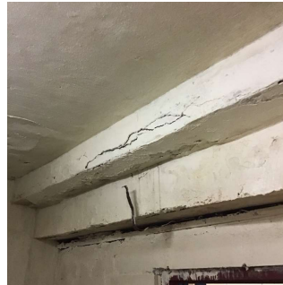
Basement - Oil Tank Room (above door)
