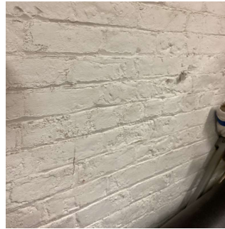
Basement - Boiler Room
