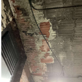
Basement - Boiler Room
