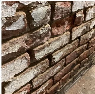
Basement - Boiler Room
