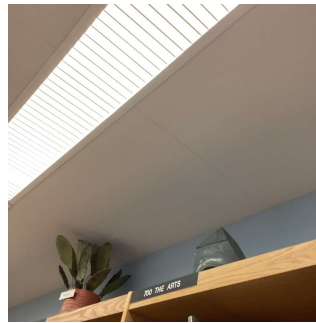
Near Room 446C
