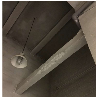
Basement - Boiler Room
