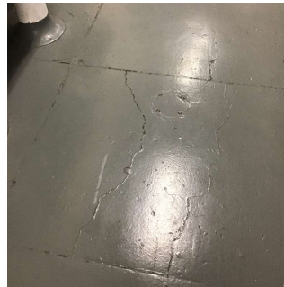
Near Drinking Fountain
