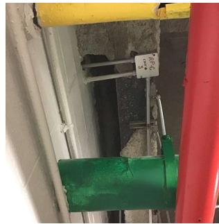
Basement - Fire Pump Room
