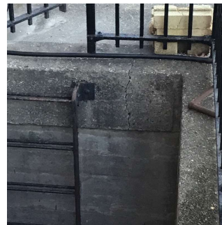
Facade A - AW2 No violations recorded.
