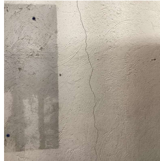
Basement - Boiler Room
