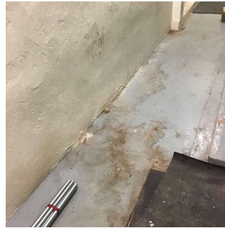
Basement - Electrical Switchboard Room B52
