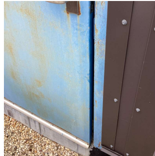
Roof 1 - Bulkhead - door does not close
