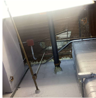
Ground Floor - Fan Room 016
