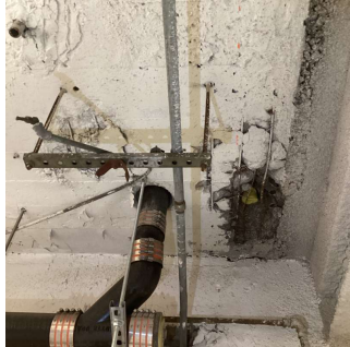
Basement - Boiler Room
