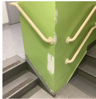
Stair C/2 (missing bottom rail)
