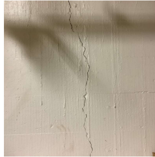
Basement - Compressor Room
