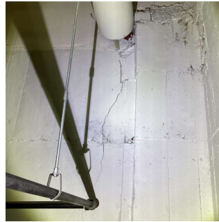
Oil Tank Room
