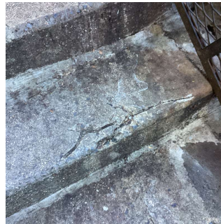
Facade A - AW1 No violations recorded.
