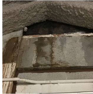
Mechanical Room Unit 6
