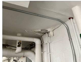
Boiler Room M203
