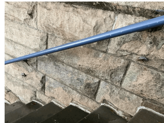
Main Entrance (children's railing missing)
