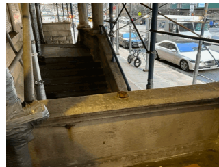
Main Entrance (railing missing on top of wall)
