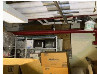
Custodian's Repair Shop C07 (boarded up)
