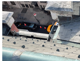
Roof 4 (loose tile in gutter)
