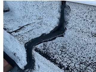
Elevator Bulkhead (damaged flashing)
