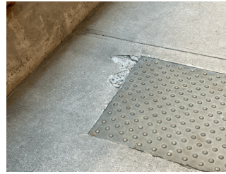
Exit 5 - HC Ramp
