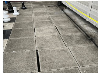
Roof 2 Plaza Deck near Metal Stair (loose pavers)
