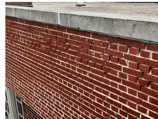
Roof 1 - Facade E (missing mortar)
