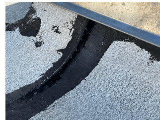
Roof 1 at Exhaust Fans
