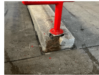
Facade A - HC Ramp
