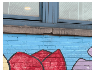
Plaza Deck - Facade F
