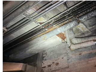
Fan Room shown, also Boiler Room
