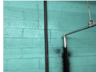
Penthouse Mechanical Equipment Room (near HV-19)
