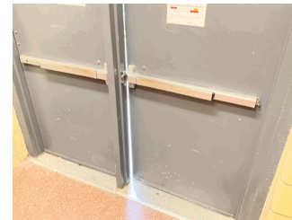
Exit 3 in Stair C (misaligned)
