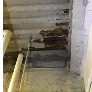
Basement - Garage near Oil Tank Room
