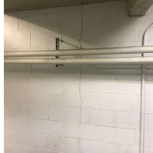
PH/Elevator Machine Room
