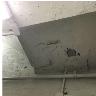
Basement Pool Mechanical Equipment Room
