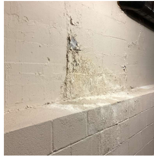
Oil Tank Room
