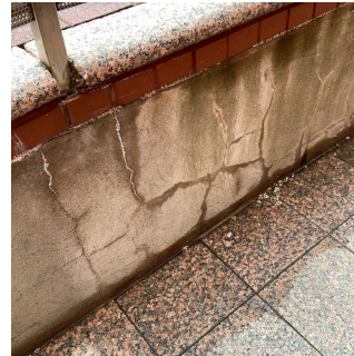
Facade A - HC Ramp
