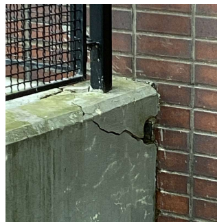
Facade A - HC Ramp
