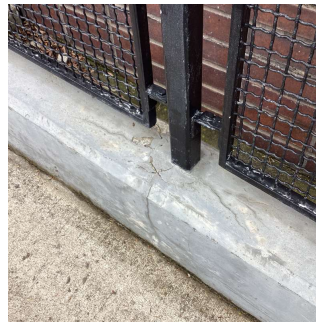
Facade A - HC Ramp
