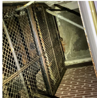
Basement - Sidewalk Elevator
