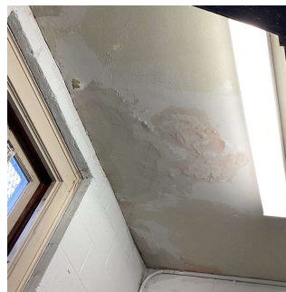
Roof 2 - 1st Floor Varsity Locker Room (Roof 2 - 1st Floor Varsity Toilet Room, Roof 1 - 1st Floor Junior Varsity Locker Room and Toilet Room similar)
