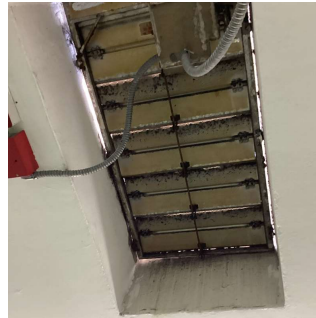
Stair A/3 - Smoke Hatch
