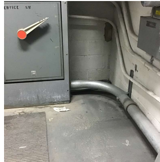
Electrical Panel Room
