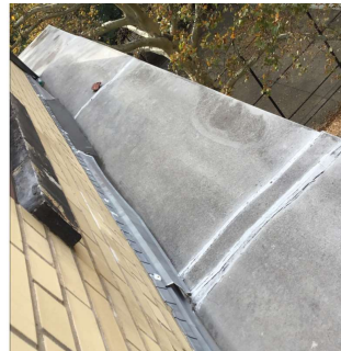
Bulk Head 3 and Coping Facade H No violations recorded.
