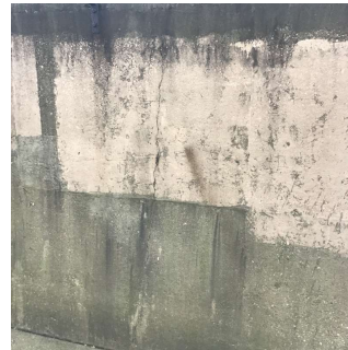
Facade A - AW8 No violations recorded.
